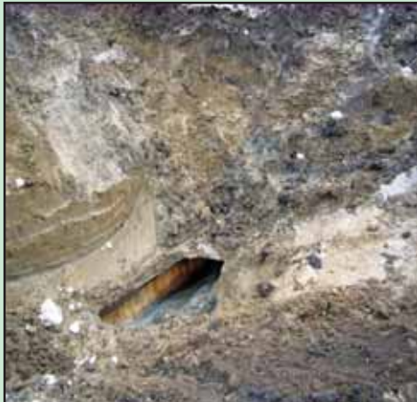
Collapsed section of 36-inch diameter wastewater forcemain
