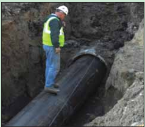
HDPE liner pipe as it is being inserted into the 36-inch diameter forcemain
