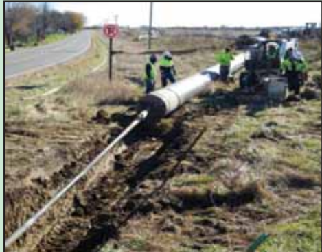
Preparing to pull a large length of HDPE liner pipe into the existing forcemain
